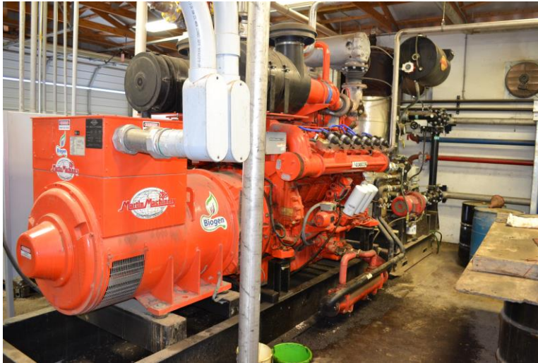
Figure 5. Guascor CHP unit
