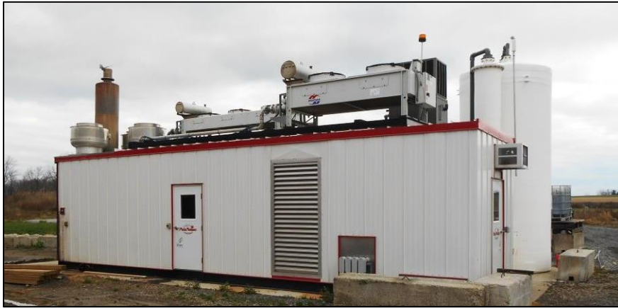
Figure 2. Combined heat and power generation skid (foreground) with adjacent H 2 S scrubber (right background).
