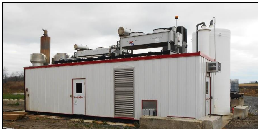
Figure 2. Combined heat and power generation skid (foreground) with adjacent H 2 S scrubber (right background).
