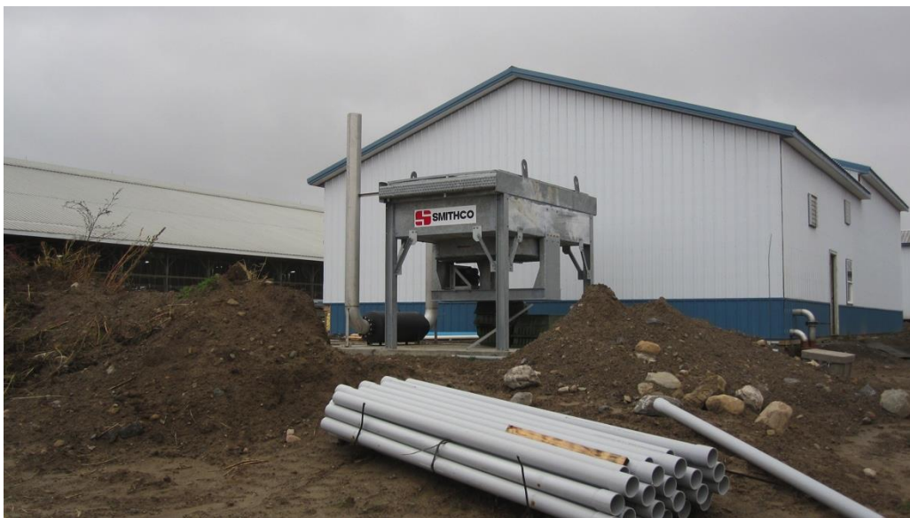
Figure 2. Lawnhurst farm biogas utilization building
