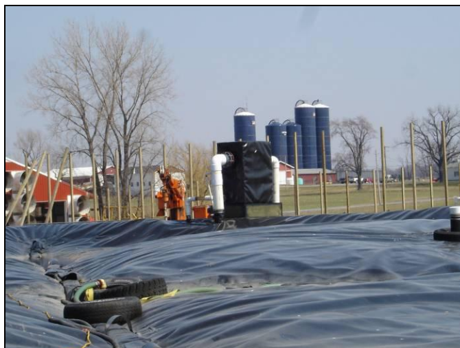
Figure 1. Patterson Farms' anaerobic digester with flexible top cover
