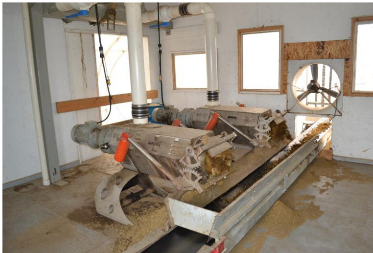
Figure 3. Solids separation room
