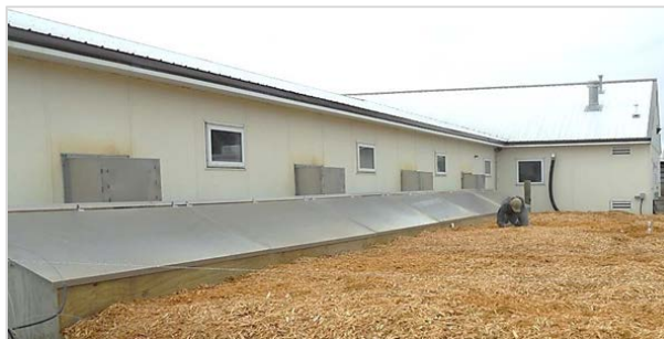
Figure 6. A low-cost, open-bed biofilter treating wall fan exhaust from a swine nursery barn.
