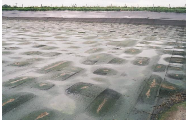
Permeable cover installed on an earthen dairy manure storage
