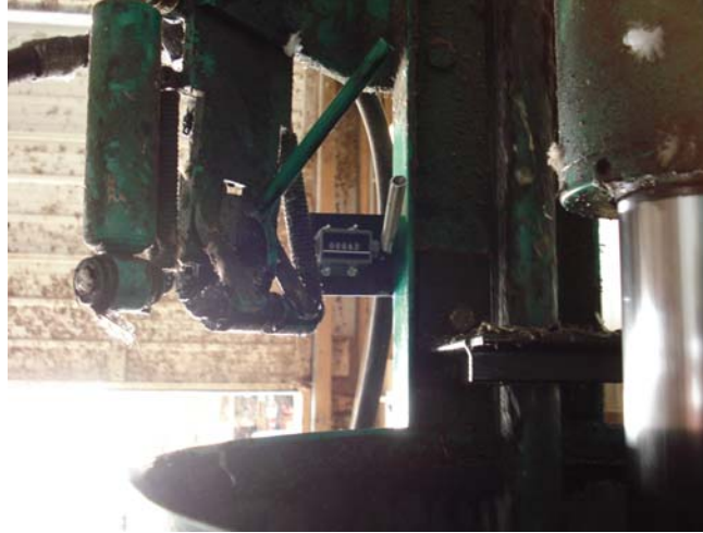
Figure 3. Mechanical counter used to track digester influent volume, installed at New Hope View Farm
