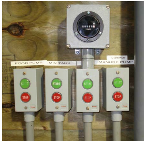
Figure 4. Patterson Farm time clock, installed to track digester influent volume.
