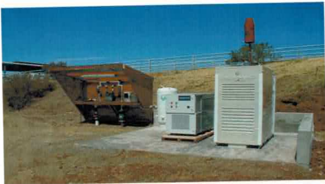
Figure 3: Biogas Handling System and 25 KW Microturbine Electric Generator
