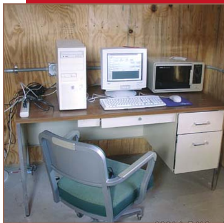
Computer control system
