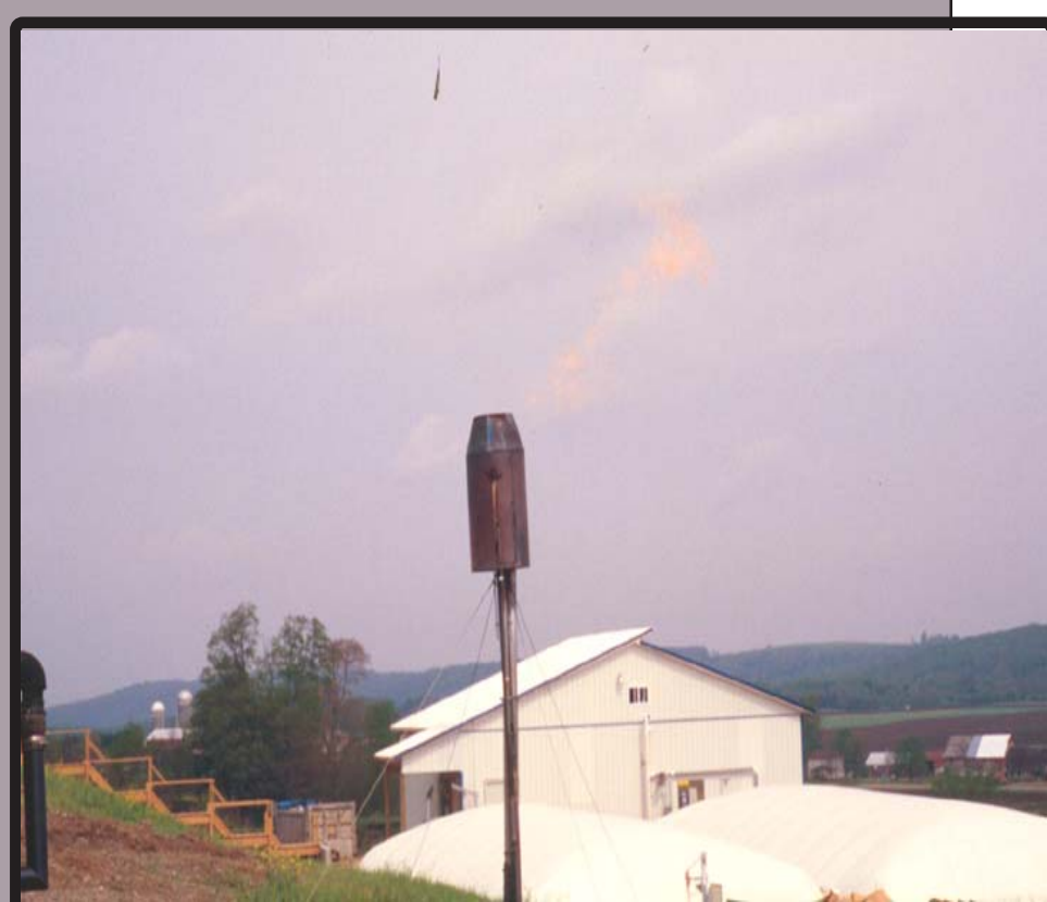
Excess biogas is flared; recently, a gas flow meter was installed to determine the amount of gas sent to the flare
