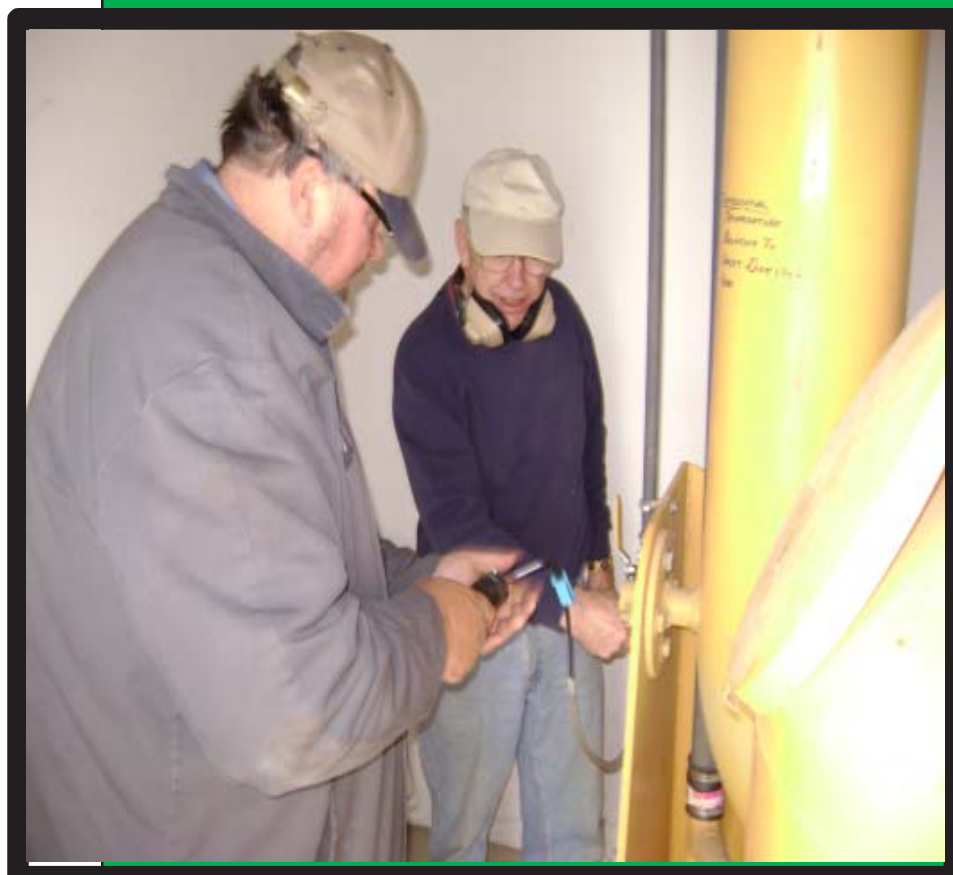
H2S testing next to gas conditioning system
