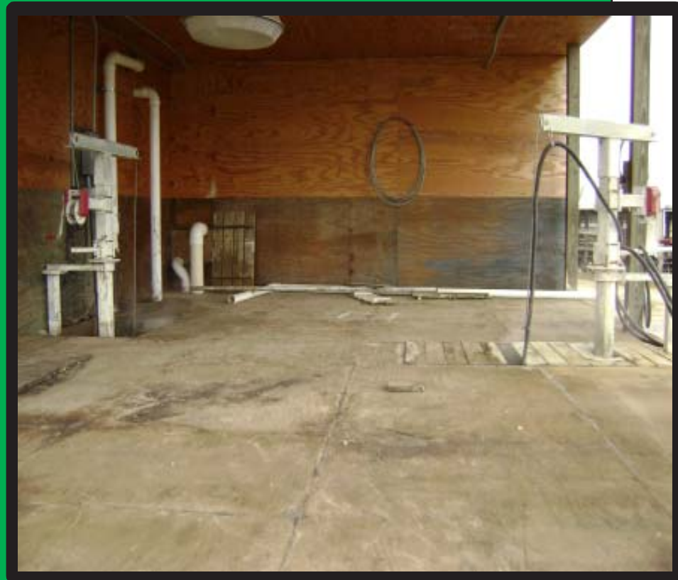
AD influent pit
