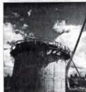
THE MANURE-TO-METHANE digester at Faber's dairy will be 35 to 40 feet in diameter and 28 feet deep - part of which which will be buried in the ground.
