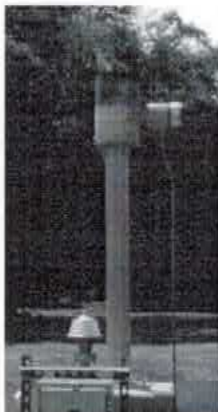
Produced at the rate of 6,000 cu. ft./day, digester biogas is currently being flared to reduce odors and methane emissions.
