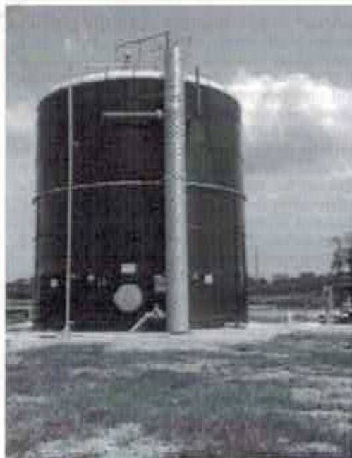
Fixed-film digesters are designed to have a smaller footprint than conventional suspended-growth digesters, an important factor where land availability is limited.
